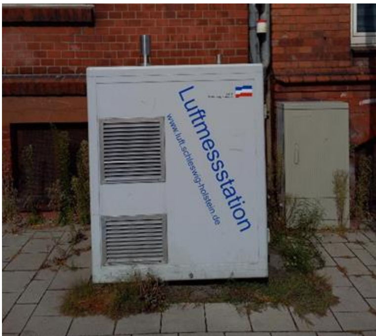
air measuring station
