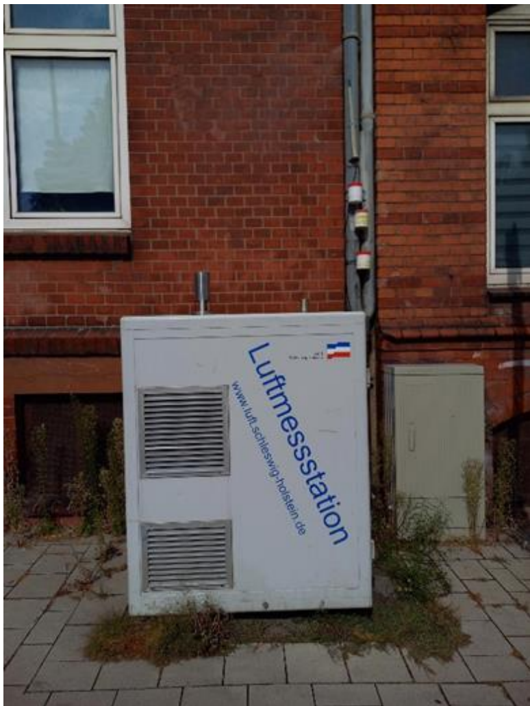
air measuring station
